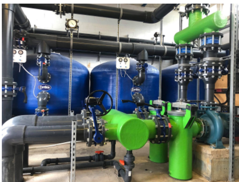
Portishead Open Air Pool's new plant system by D & G Pool and Leisure Ltd
