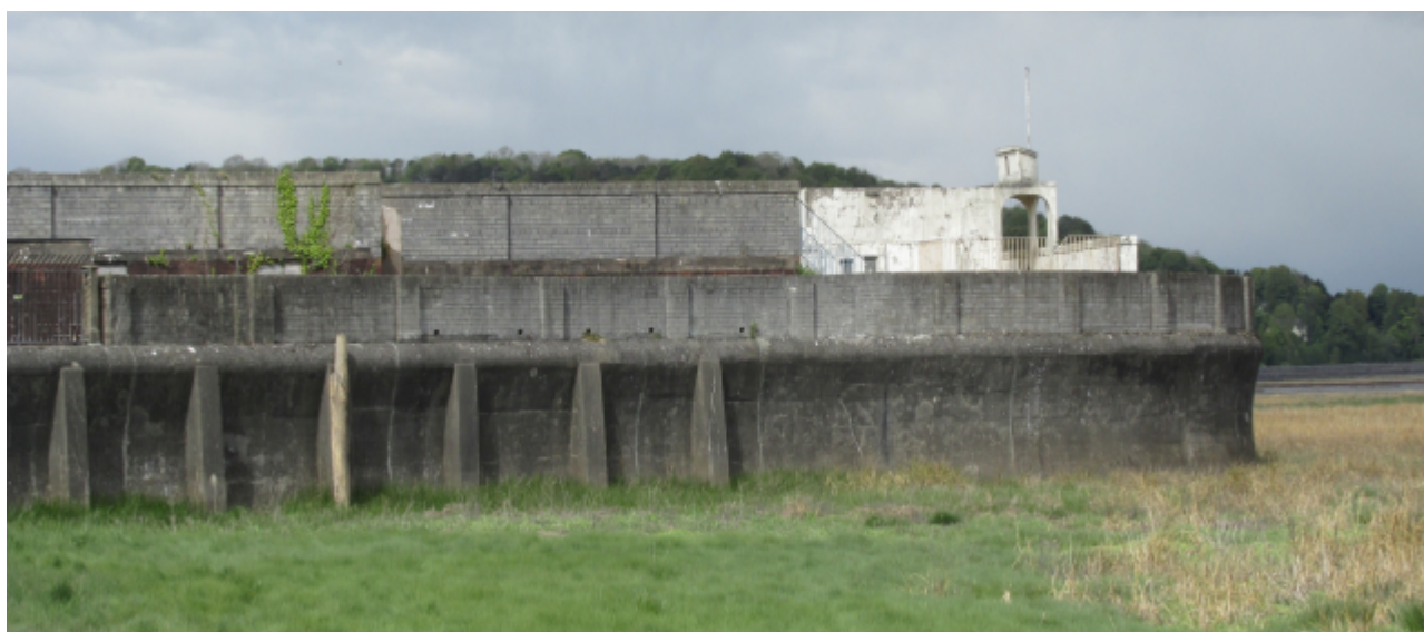
The outer wall of the Lido forms part of the sea defences for Grange
